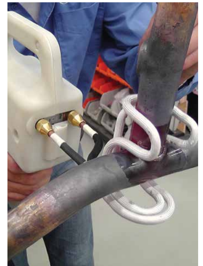
5. The UBraze is re-positioned on the other side of the joint, to heat the area previously left open by the T Coil.
